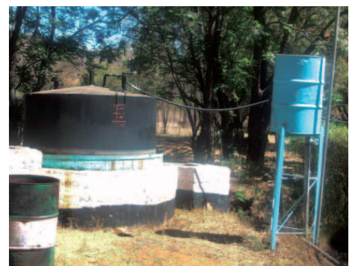
Gas collection tank resting on the concrete-built digester. Pipes / tubes at the top of the gas tank supply the house with methane gas, Botswana. (Reuben Sebege)
