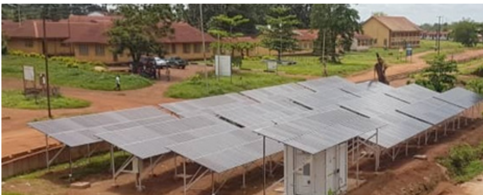
Installed solar Pv System
